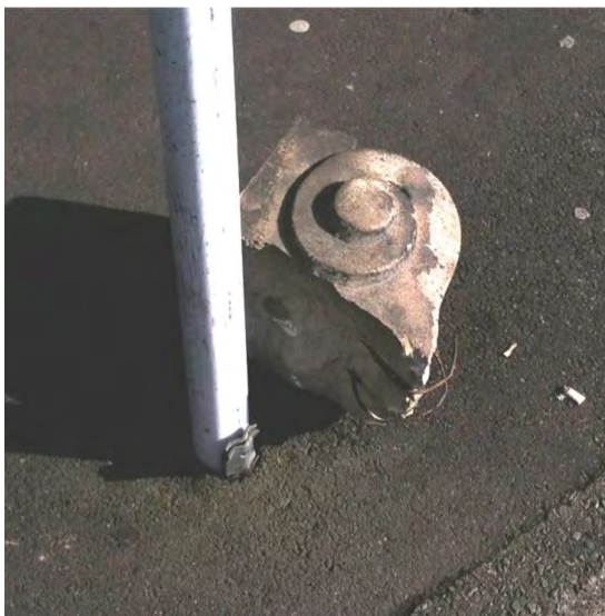
This concrete corbel fell from a Wellington building in 2013. Photo: Wellington City Council, 2013
