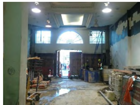
The former Evening Post building on Willis Street was earthquake-strengthened in 2014 with help from the Built Heritage Incentive Fund (now HRRF). Image: Wellington City Council.
