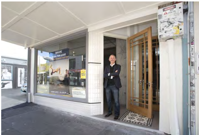
216 Cuba Street received funding from the Built Heritage Incentive Fund to help develop a detailed seismic strengthening scheme and complete the strengthening works. The work included installing concrete moment-resisting frames so the shop display window is not obscured. Photo: Wellington City Council
