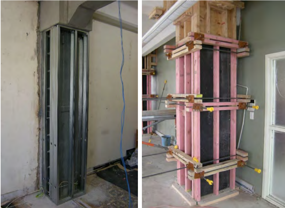
15 Courtenay Place is an example of a building where the performance of the existing structure has been improved. The image to the left shows continuous columns installed through the whole building from the ground floor to the top of the building. While the image on the right shows Continuous steel jackets installed around four of the existing columns from the ground through to 600mm above the floor on level 4.
