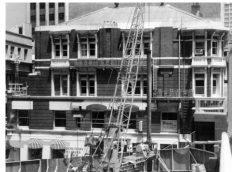
This photograph shows 97 The Terrace in 1978. The original corner turret may have been removed after the 1942 Wairarapa earthquake. The building has recently been strengthened. Image: Charles Fearnley, Wellington City Recollect 50003-1301
