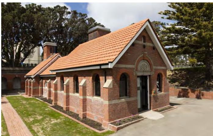
New pattress plates have been installed to secure the gable end of the Karori Crematorium and Chapel. Pattress plates (sometimes called rosettes) are a traditional feature of old brick buildings and are usually painted black. Photo: Neil Price, Wellington City Council.
