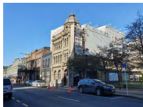
The Albemarle Hotel is being strengthened with help from the BHIF. Photo: Moira Smith, 2022
