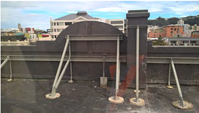
New structure has been installed to secure the existing chimney and parapet for the former Cadbury building. It is not visible from the street. Photo: Wellington City Council.
