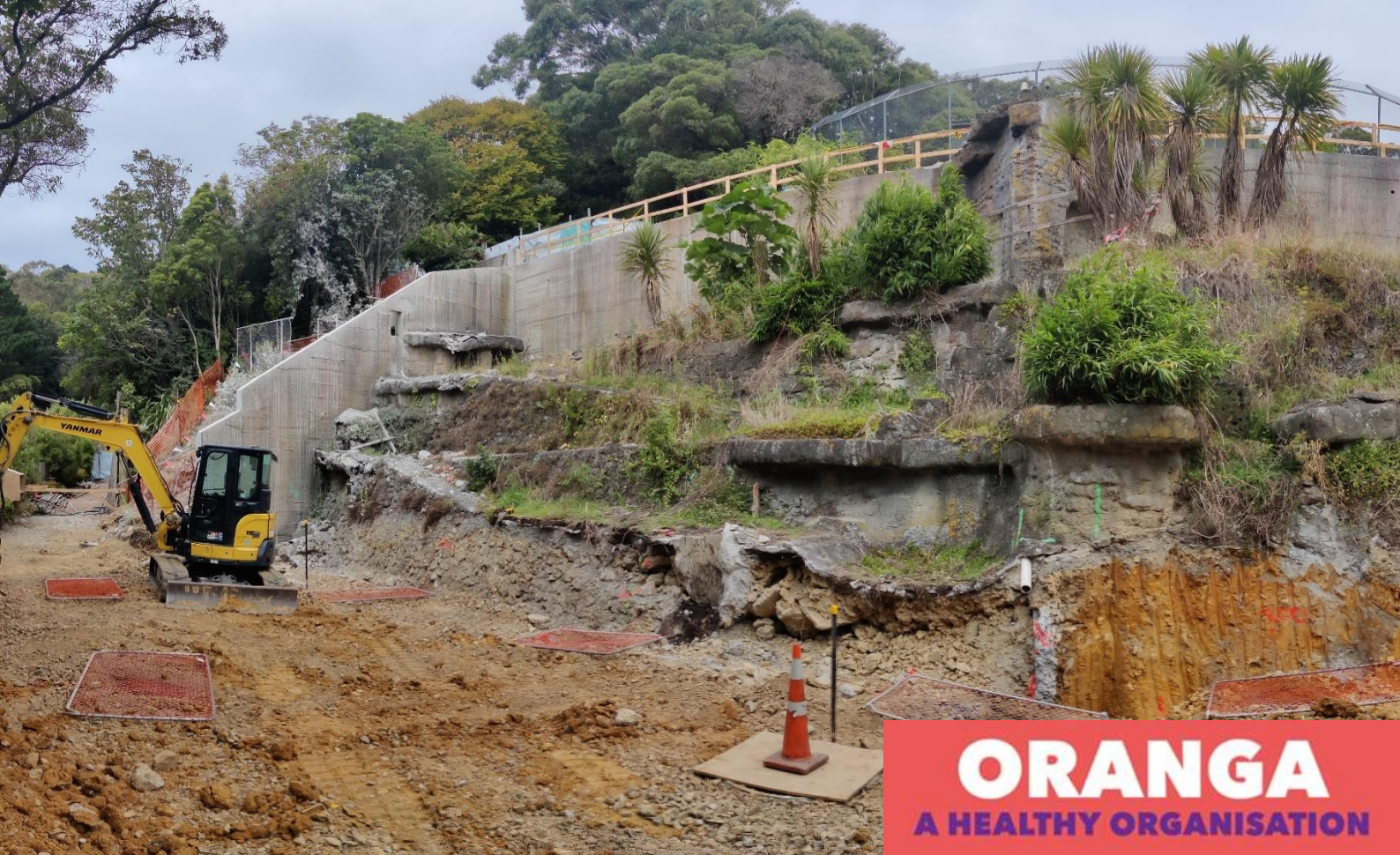
Photo: Demolition of new Snow Leopard site as at end of February (C Jerram)
