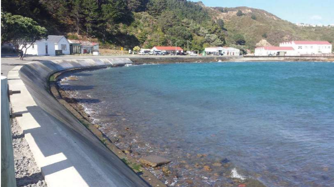
The Northern bay showing recently treated sea wall area (foreground) and untreated sea wall area in distance
