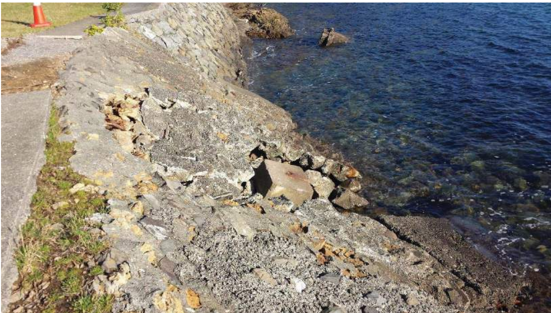
Damaged area of Southern bay
